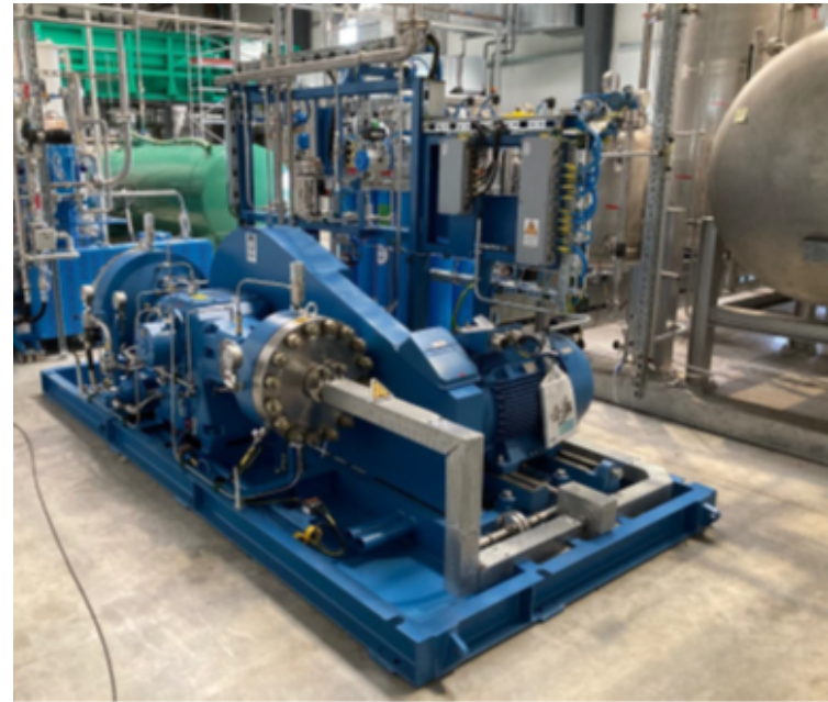
Figure 7: H 2 compressor. Credit: Fraunhofer UMSICHT.
